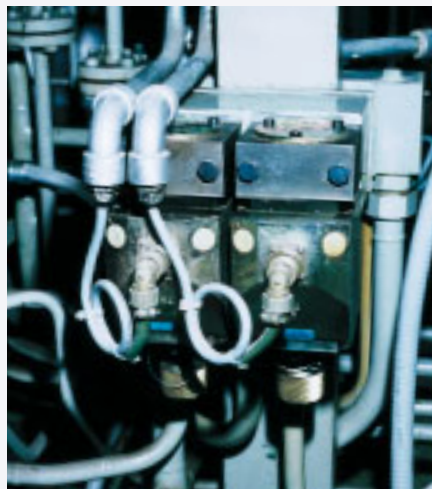
A typical installation in a cogeneration plant.
